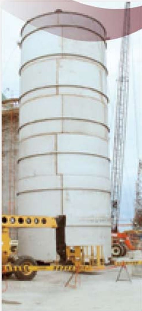
Storage tank • Quebec, Canada
