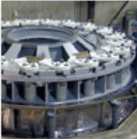
Turbine • Chamera, India
