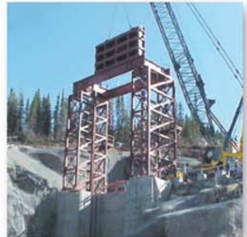
Dam Gates • Quebec, Canada
