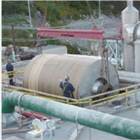
Installation • Quebec, Canada
