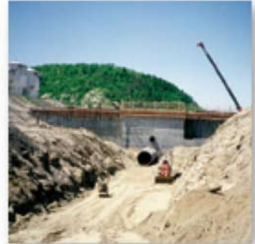
Underground Piping • Quebec, Canada
