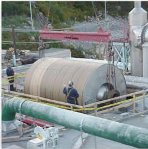
Installation • Québec, Canada
